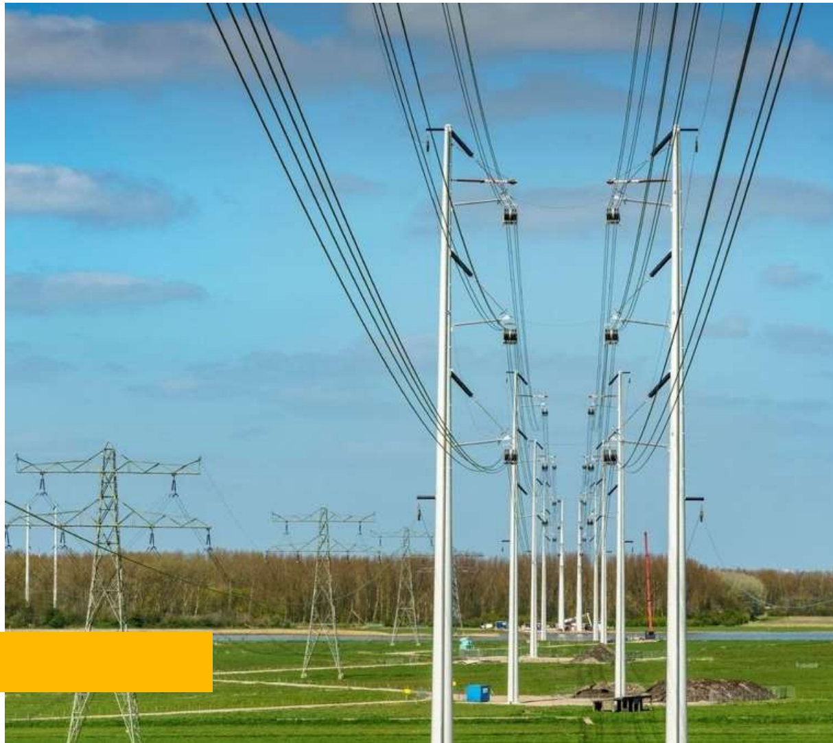
WINTRACK II - TENNET INFRA
